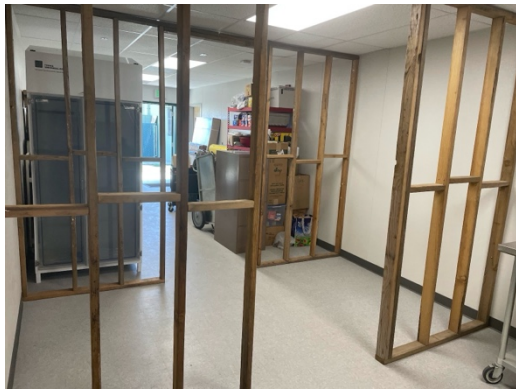
Four individual walls were constructed in the woodshop and then installed onto the room walls.
