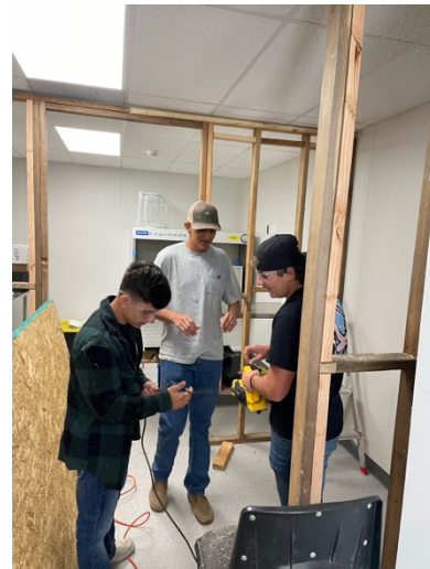
Students using a battery power planer to ensure all 2x4s are flush with one another prior to installing the plywood over the top
